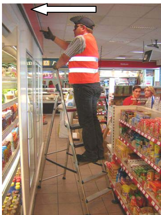
Shot shows display panel area and position of ladder
